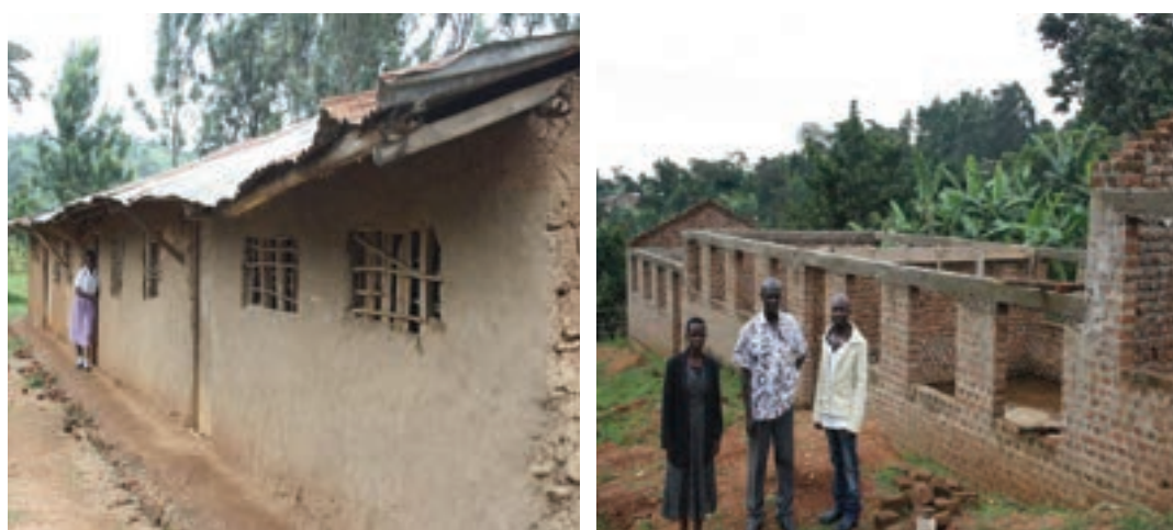
Figure 3: A temporary classroom block at Buzalangizo P/S and a new classroom block on the right being constructed at the same school
