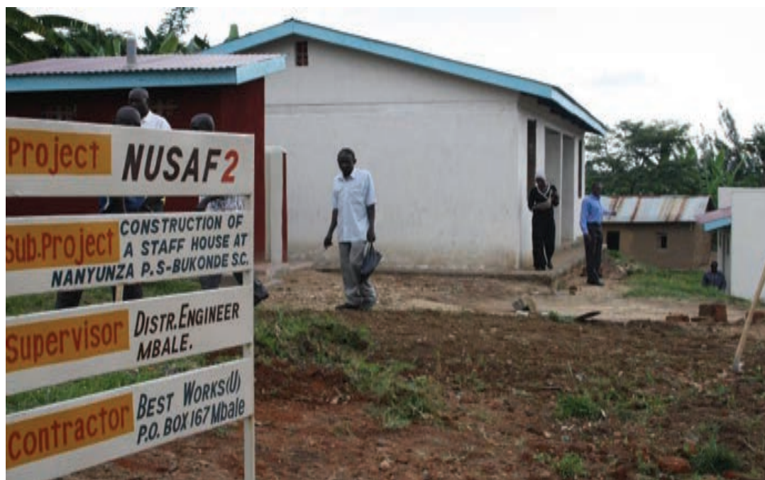
Figure 4: A new teachers' house being constructed at Nanyunza Primary School, Bukonde Sub-county under the NUSAF 2 Project
