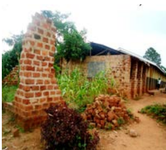
Figure 11: The only concrete classroom block at Kikunyu COU PS. The block has remained incomplete for over three years.
