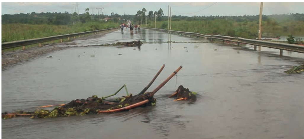
Mbarara Masaka Highway cut off by flash floods at Katonga Bridge, May 2023.
